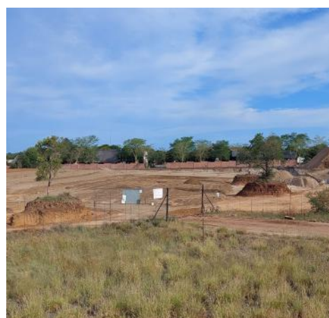
The "Fire Station" entrance to the building site of the Maruleng Mall. Image supplied
